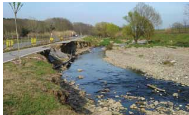
Erosion has undermined this cycle path and now threatens the safety of the adjacent road.
