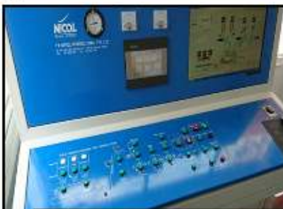
MODERN CONTROL PANEL
